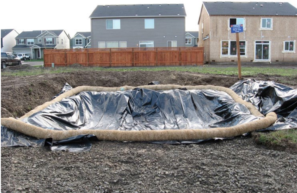
BEST MANAGEMENT PRACTICE: THIS CONCRETE DISPOSAL AREA IS CLEARLY DEMARCATED, LARGE ENOUGH, AND CONSTRUCTED BELOW GRADE TO MAXIMIZE CONTAINMENT.
